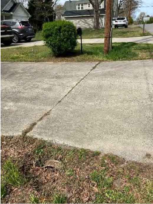
Photo 5: West side of Grace Avenue looking North – Clogged pipe under driveway at 505 Grace Avenue full
