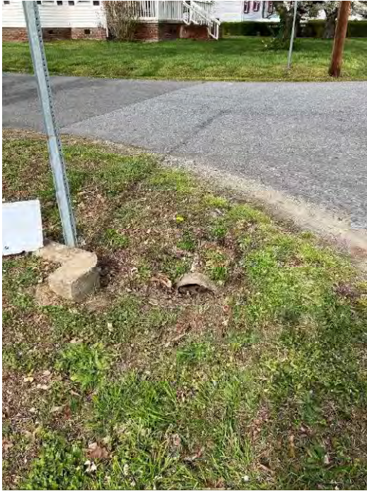
Photo 5: Southwest corner of Cook Street and Cadillac Street – Clogged outlet pipe
