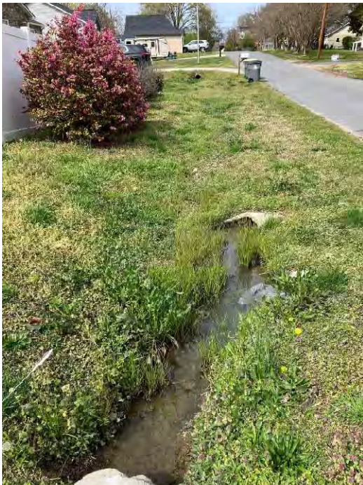
Photo 7: West side of Marie Avenue looking northeast – Ponding at double barrel inlet
