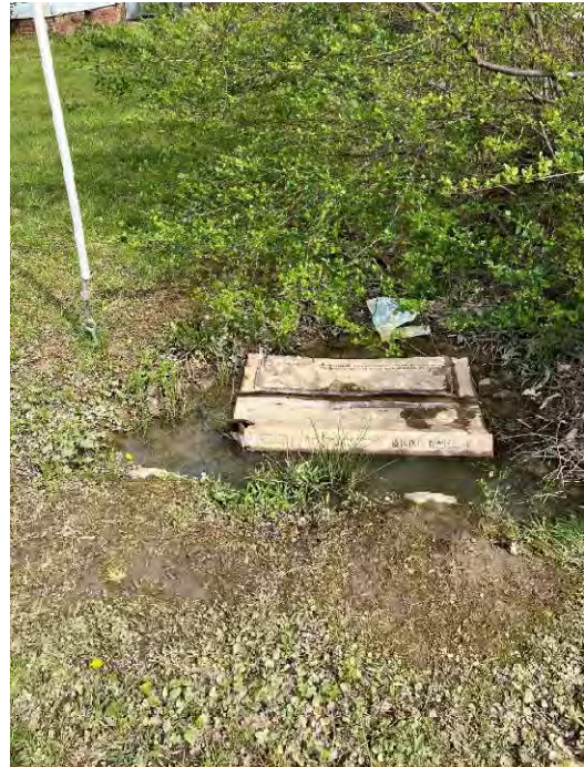
Photo 6: West side of Marie Avenue looking east – Ponding at double barrel outlet
