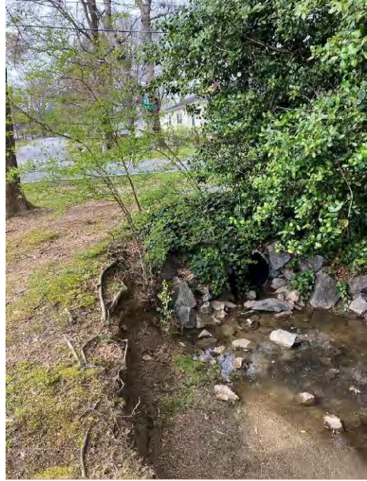
Photo 2: Looking north from south side of Cook Street – System outlet
