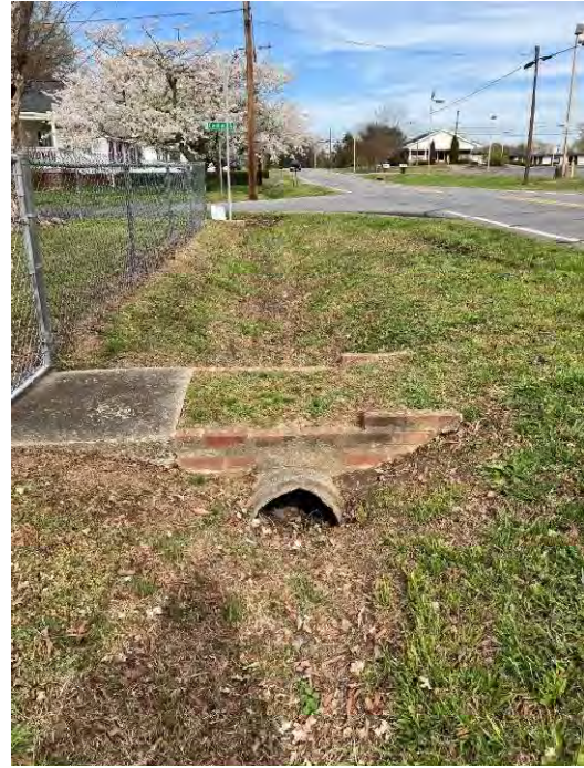
Photo 6: North side of Cook Street looking east – Clogged outlet pipe
